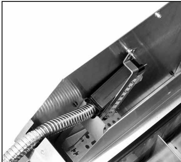
SMHA-4 with top cover removed and soda manifold installed.
